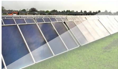
Solar district heating
