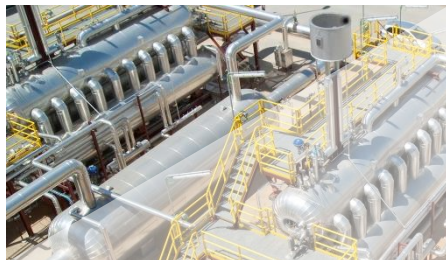
Header-coil heat exchangers
